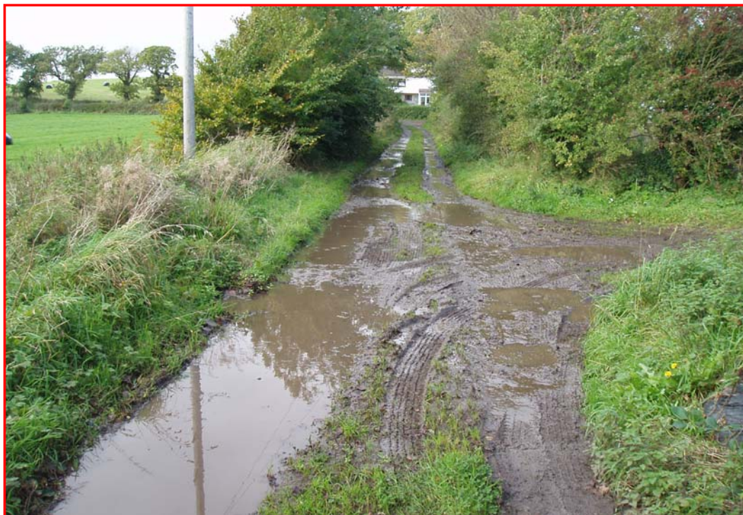
Access Road Flooded
